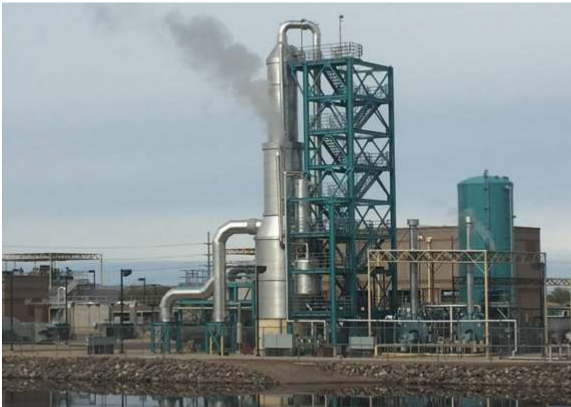
Figure 2-3 Concentrate Evaporator Rated for 250 gpm at a Facility in Chandler, Arizona
