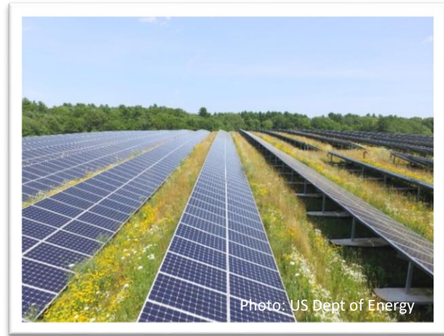
Solar farm built on a landfill in Rehoboth, MA.
