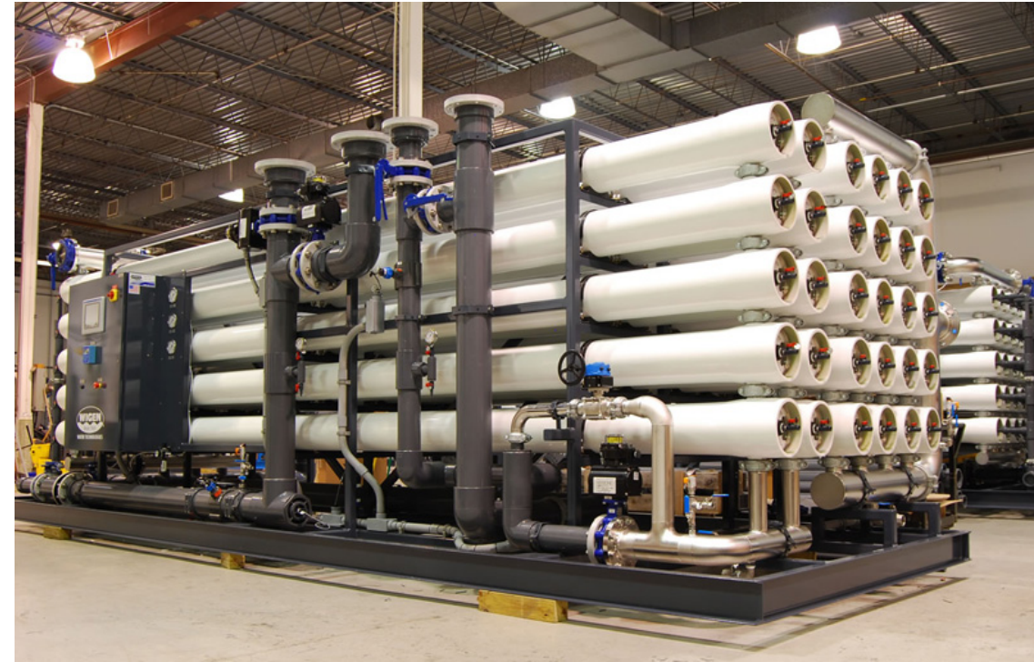
Drinking water plant reverse osmosis membrane skid
