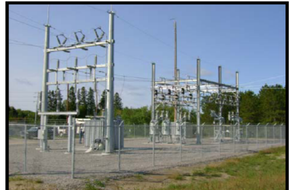
Typical 115 kV Distribution Substation
