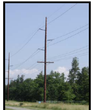
Typical 115 kV Transmission Line With Distribution Underbuild
