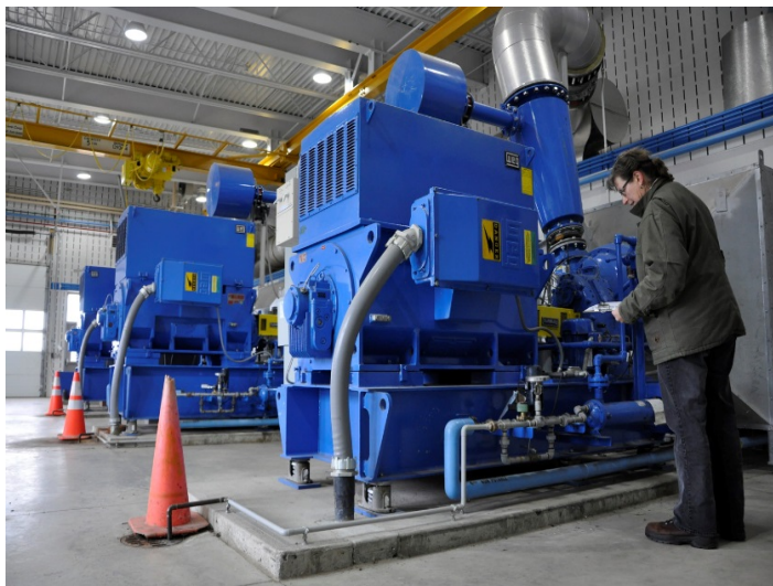
Auxiliary equipment provides backup service at MCES wastewater treatment plants during floods, power outages, and other emergencies. Source: Metropolitan Council
