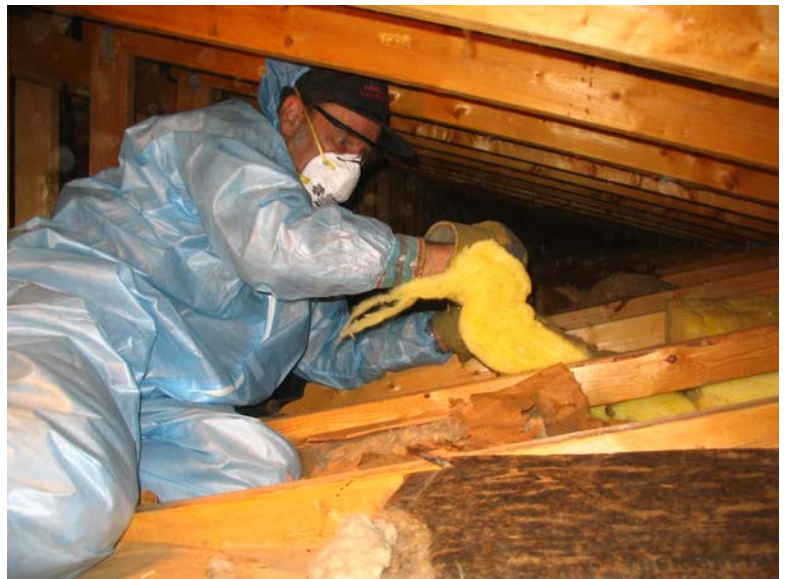
Adding batt insulation in the attic reduces heat loss and increases energy efficiency. Photo from the Minnesota Department of Commerce
